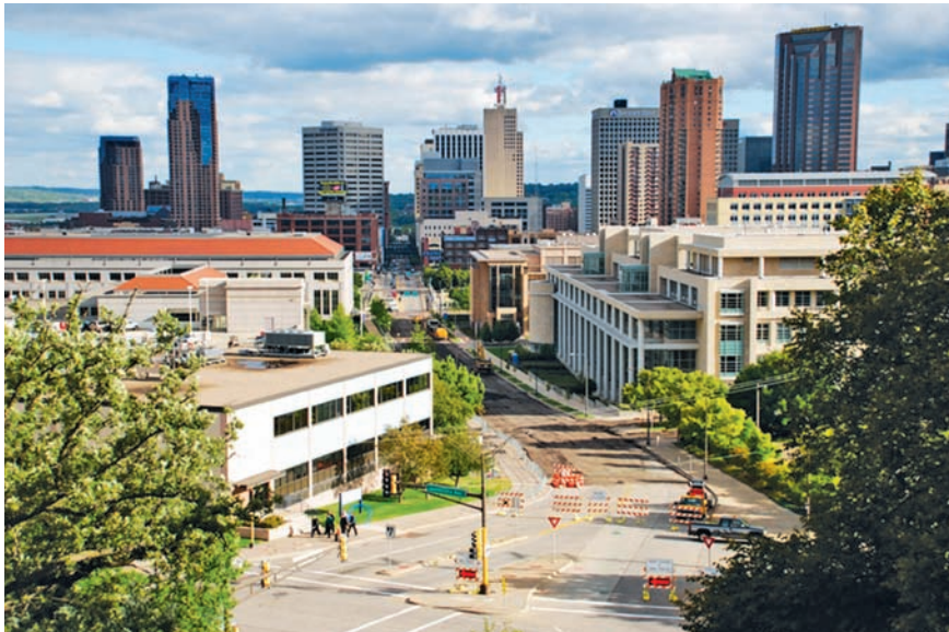
St. Paul: Robert Street's surface is removed between University Avenue and 12th Street, the first day of construction, September 7, 2010, on the Central Corridor LRT.
